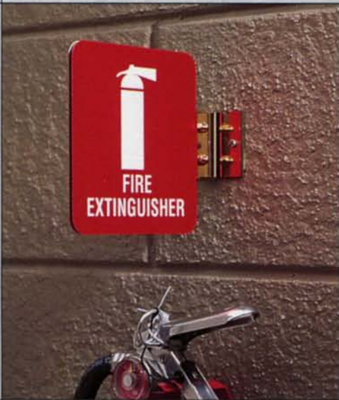
Fire Equipment Signs
