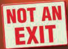
Not An Exit Sign
